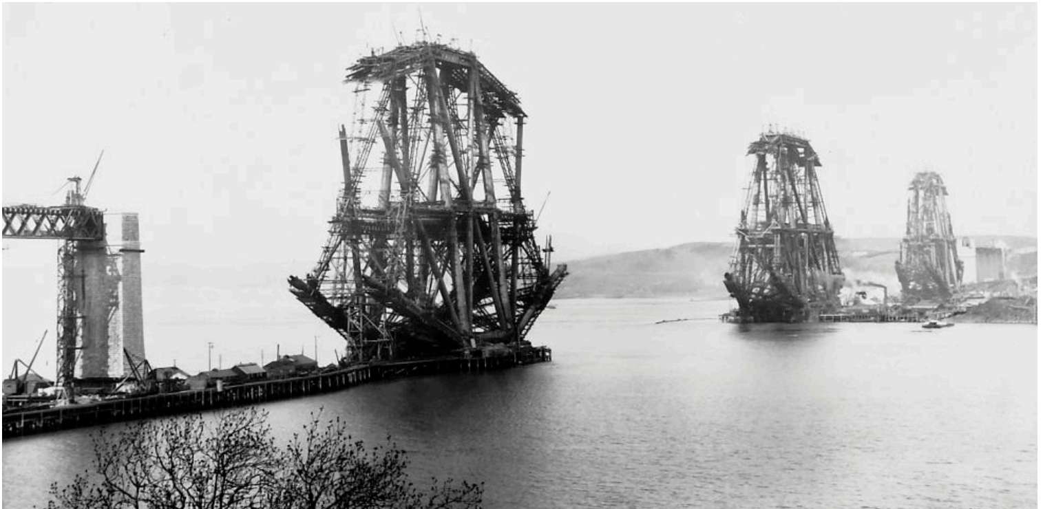
The Forth Bridge , Scotland, south approach viaduct girder-span and end pier in construction, the central towers of the three piers are at full height and the double cantilevers under construction, 10 May 1888. Crown copyright. National Records of Scotland, BR/FOR/4/34/299
